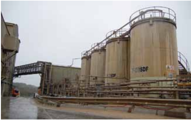
Figure 1. Steetley Dolomite's Thrislington dolomitic lime plant faced challenges in burning SDF prior to oxygen injection.
