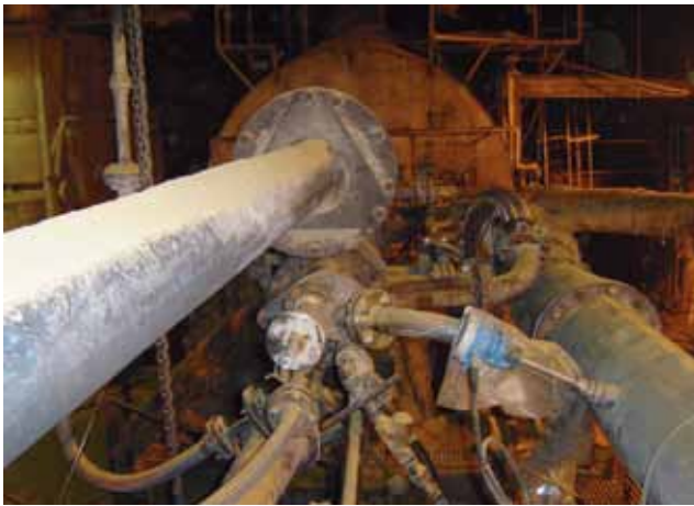
Figure 2. Air Products engineers designed the oxygen system as an easy retrofit.
